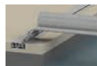
Flush mount rail in the pool surround
